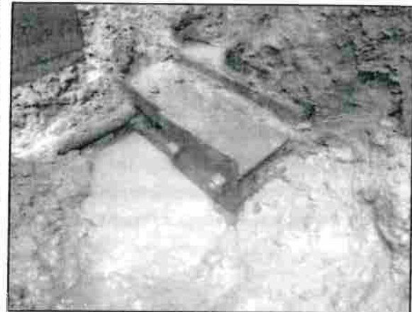
Photo 4.2-6: Steel double channel wale with moderate corrosion and section loss.
