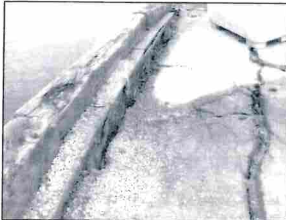
Photo 4.1-11: Observed sinkhole extents on 6/5/2019.
