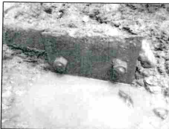
Photo 4.2-5: Steel bearing plate and through bolts with minor corrosion.
