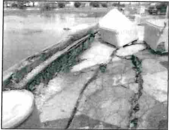
Photo 4.1-14: Observed loss of fill and sinkhole depression on 6/11/2019.
