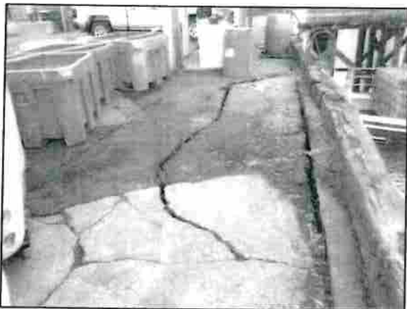
Photo 4.1-7: Additional settlement of the pavement observed at the back of the sheet pile wall.
