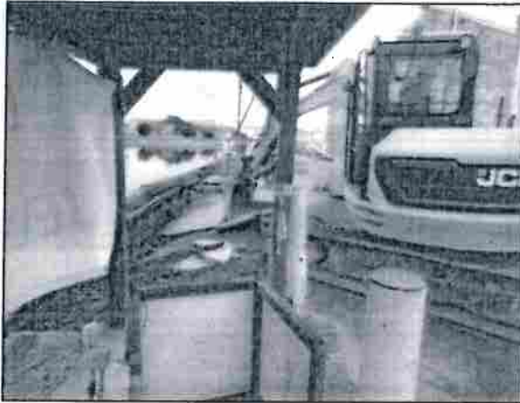
Photo 4.1-17: Removal of failed asphalt and concrete slab above the sinkhole.
