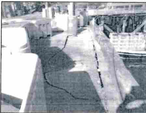
Photo 4.1-1: Deterioration observed at the top of the wall
